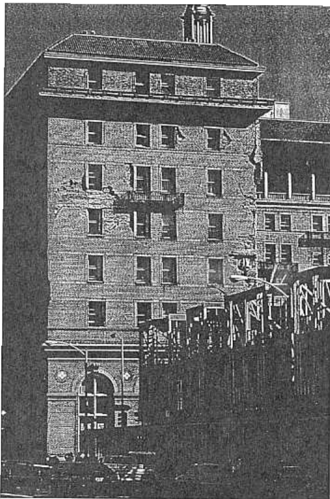
THE REMOVAL, PRIOR TO THE LOMA PRIETA QUAKE, OF INTERIOR MASONRY PARTITIONS FROM THE HOTEL OAKLAND MAY HAVE CONTRIBUTED TO THAT STRUCTURE'S DAMAGE. WITHOUT THE PARTITIONS, ALL OF THE LOADS HAD TO BE CARRIED BY THE REMAINING MASONRY OF THE EXTERIOR FACADE. PHOTO BY RANDOLPH LAGENBACH.
